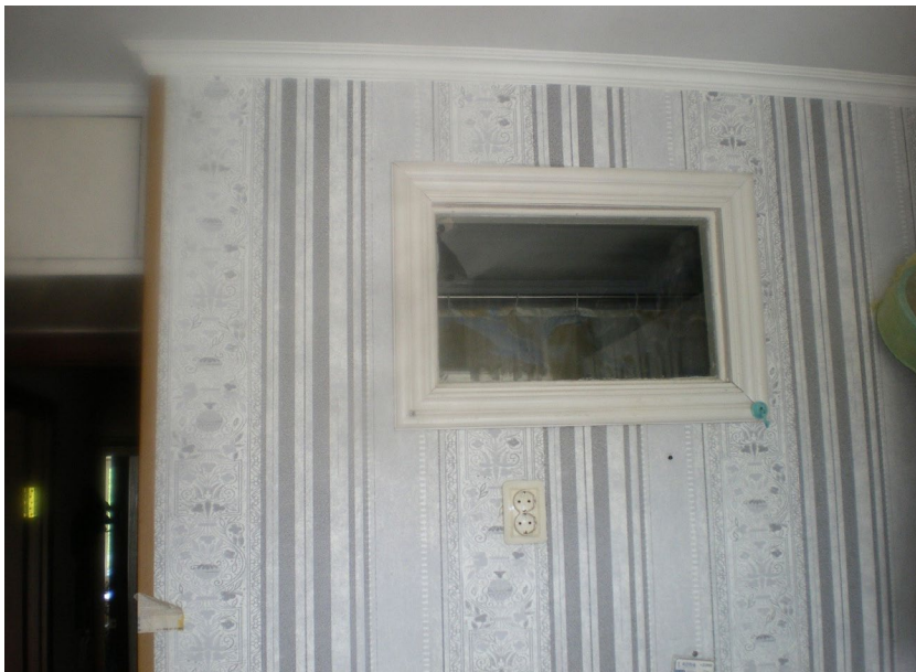
Figure 2. Position of window in bathroom from the kitchen side. Photograph by Alexander Kim.
